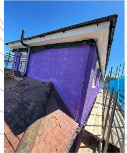
5.1.4 Preparation work on a retrofit before the application of Passive Purple External.
